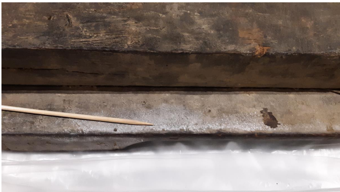
Fig. 3 Underside of proper right door 1993.1.14b. Location of Sample 2 shown with skewer
